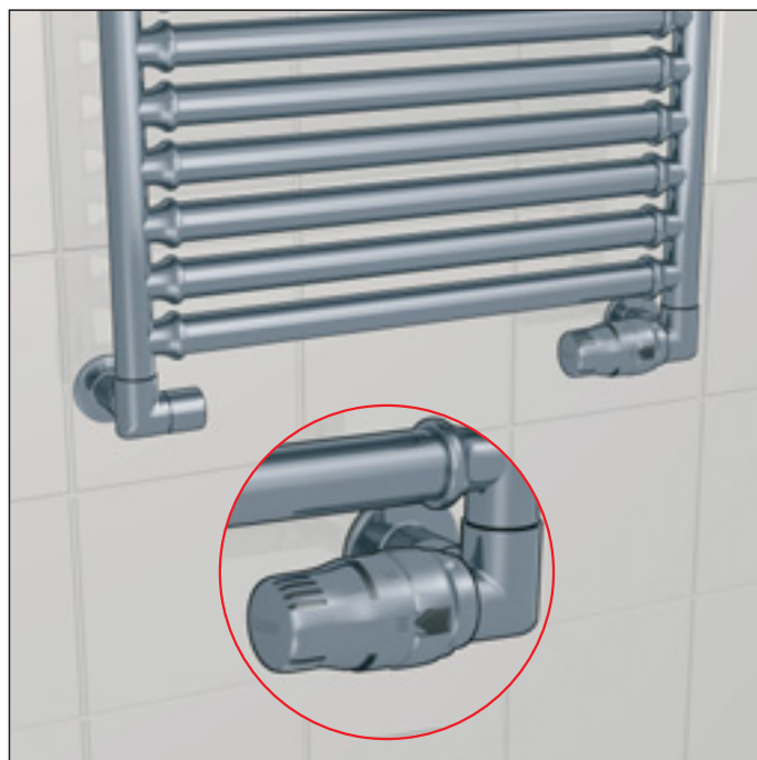
Example of high-style valve installation for designer heating systems with thermostatic control
